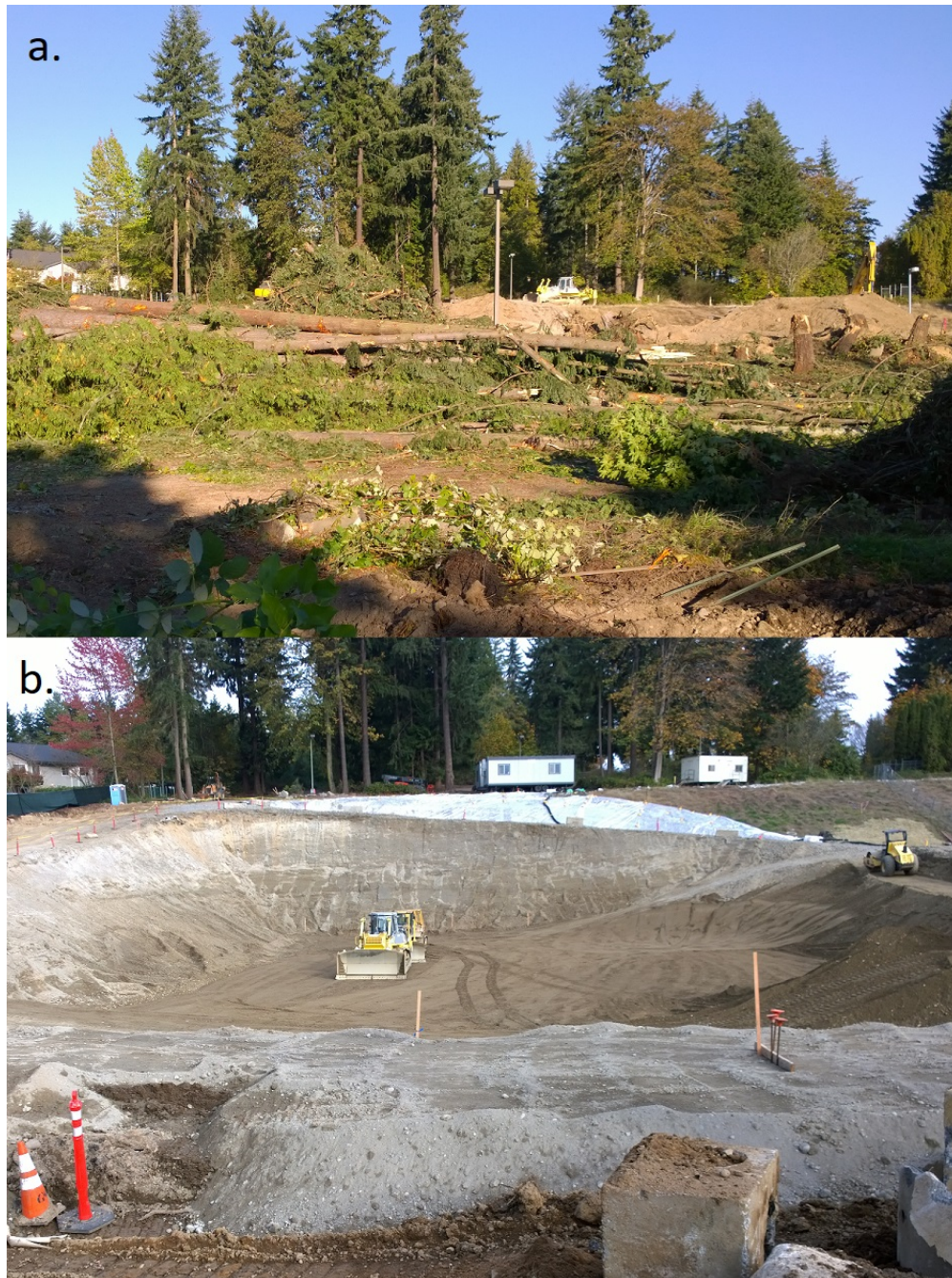
Figure 2.1: Time series of a commercial development project located in Redmond, WA showing typical tabula rasa style development where all vegetation and topsoil is removed or altered. a. Clearing the site of vegetation. b. Grading the site and digging foundation. Photos taken by the author four weeks apart in 2015.
