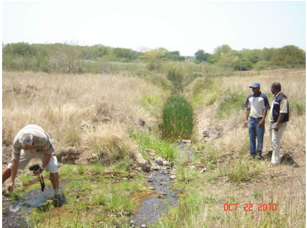
Photo 1: Seepage at the northern end of the dam wall.
