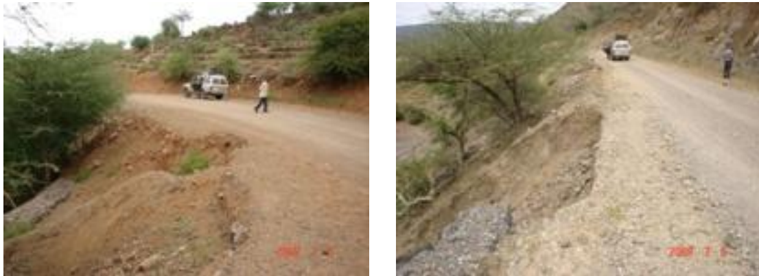
Photo: Shows road slide between km 11 and 15, which require construction of retaining wall
