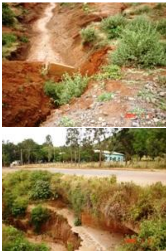
Photo: Erosion at the downstream of culverts due to concentrated flow at about km 77 and 100
