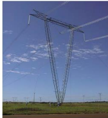
SUSPENSION TOWER - GUYED V TOWER
