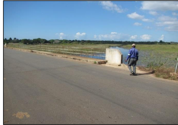
Figure 75: The double lane R241 Inhassoro road as it crosses the Govuro River in 2018
