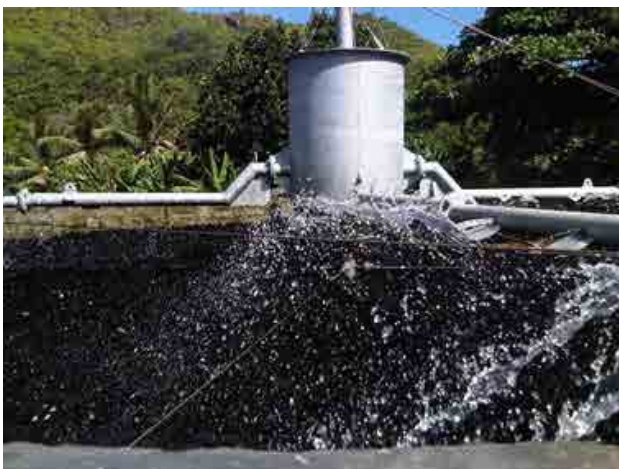
Organically loaded (dirty) water being sprinkled over the bioballs in a trickling filter.
