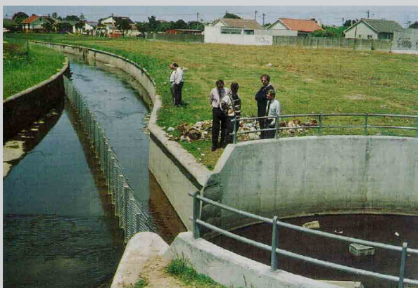
Enviroscreen installed at the Vygekraal Canal (Armitage et al. 1998)
