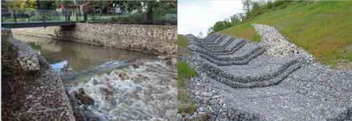
Example of a hydraulic drop installed along a river to control the river's gradient and the carrying velocity of particles.
