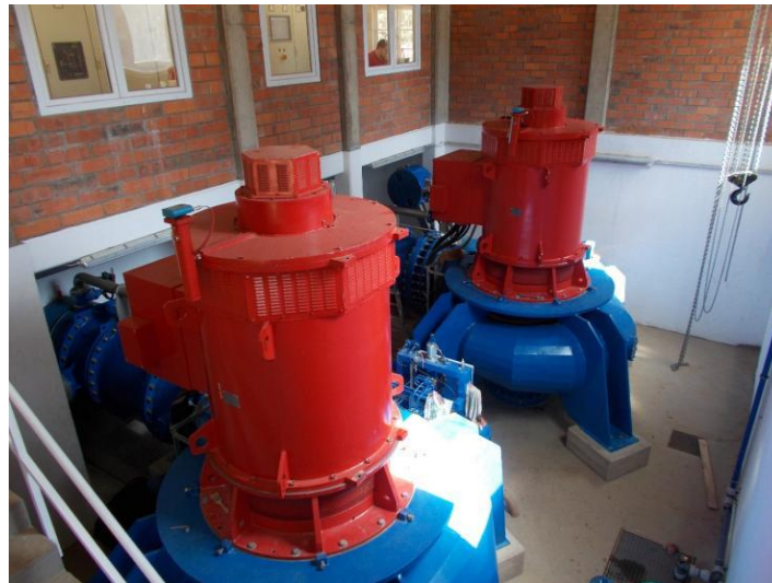
Figure 18. Example of 2 vertical-axis Francis sets
