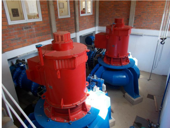
Figure 20. Example of 2 vertical-axis Francis sets
