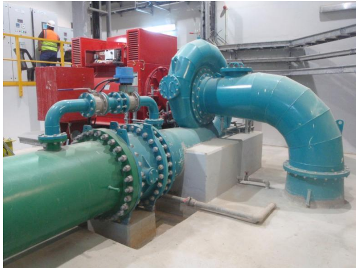
Figure 17. Example of horizontal Francis set
