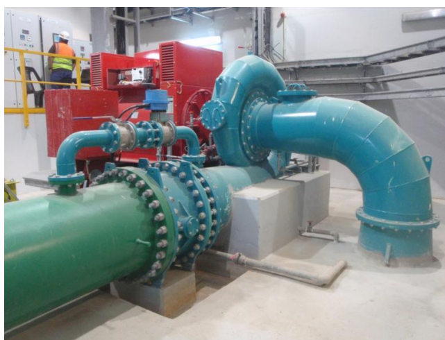
Figure 17. Example of a horizontal axis Francis set
