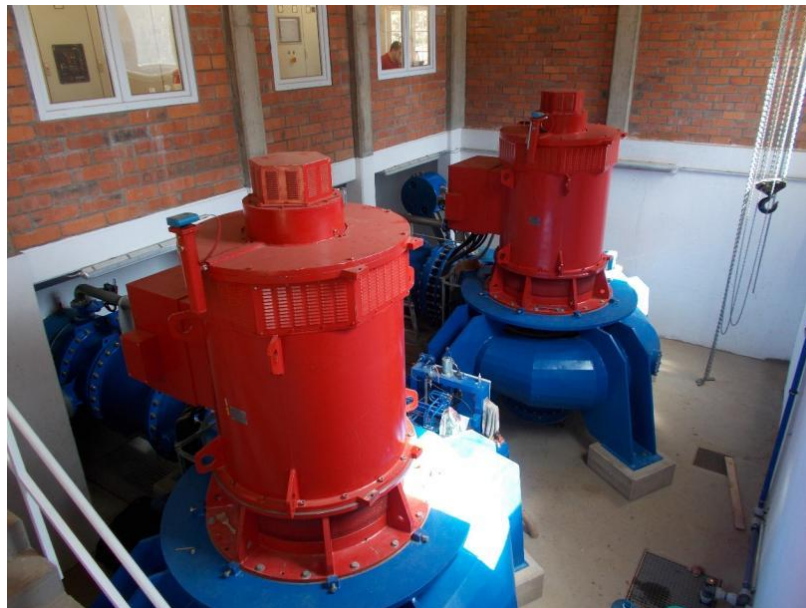
Figure 17. Example of vertical-axis Francis sets
