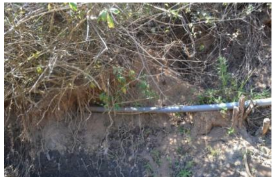
Water distribution system (PVC pipe)
