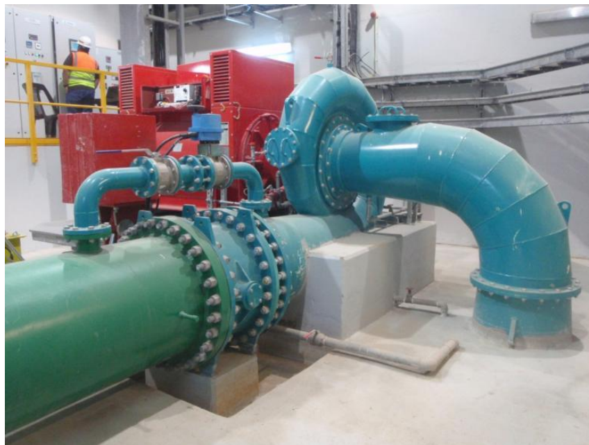
Figure 20. Example of a horizontal-axis Francis set
