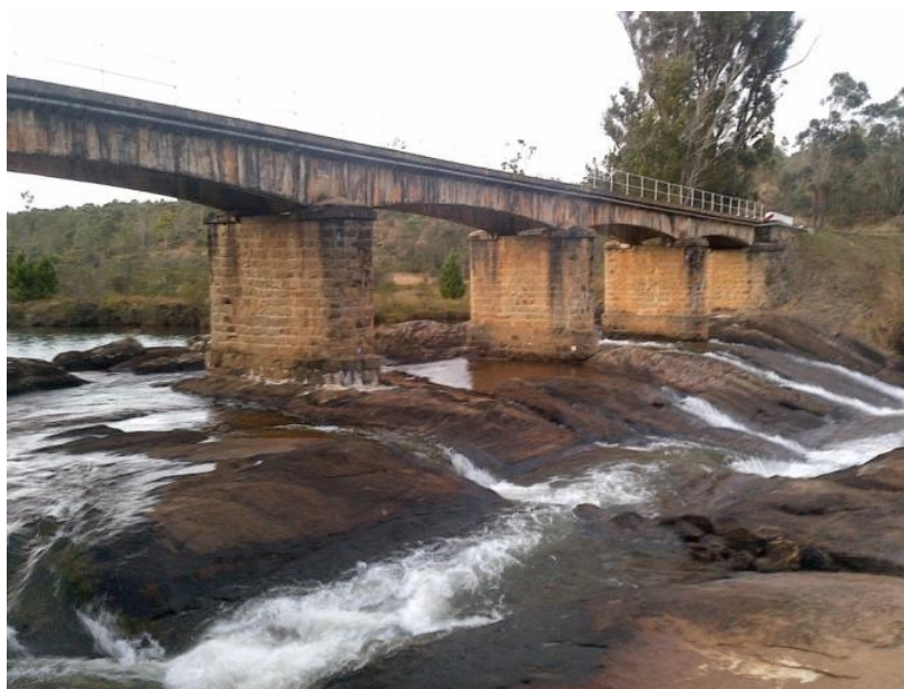
Figure 3: Upstream stretch of the rocky outcrop that creates the waterfall, where the bridge is based
