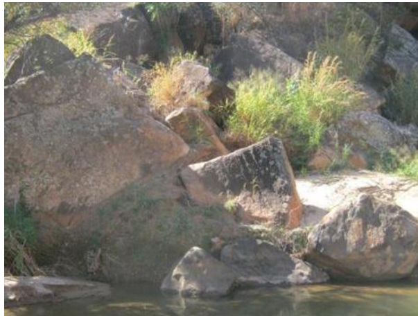
Figure 14. Boulders not in place on the right bank of the proposed weir axis
