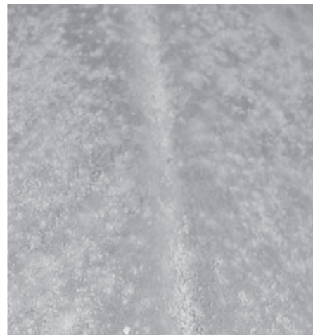
B. Close up view of rust
