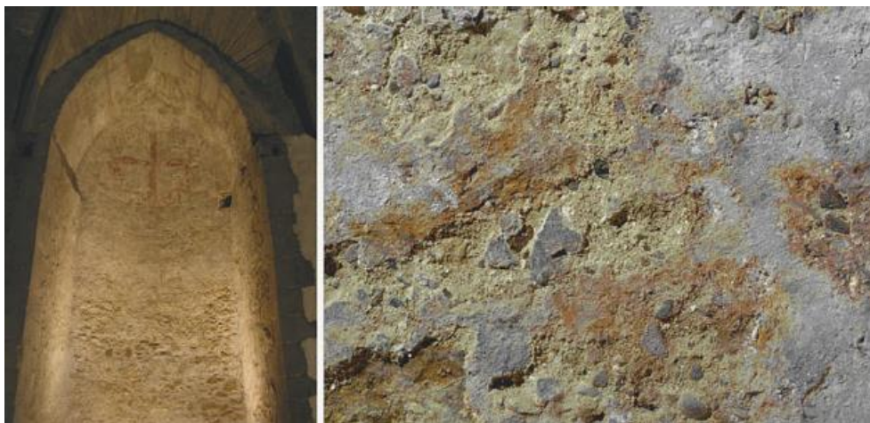
Figure I-16. Rosy stain on the salt damaged stone surface of a Medieval monument, Austria, promoted by halophilic bacteria and archaea (Siegesmund and Snethlage, 2011).
