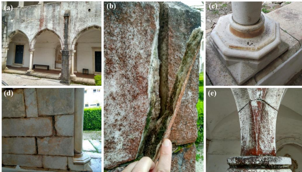
Figure V-3. Some of the pathologies found in the main cloister of the Convent. Dark staining on column stems (a), reddish staining with detachment of the material (b and e), and patina formations on the Tuscan pillars (c) and on the stone walls (d).
