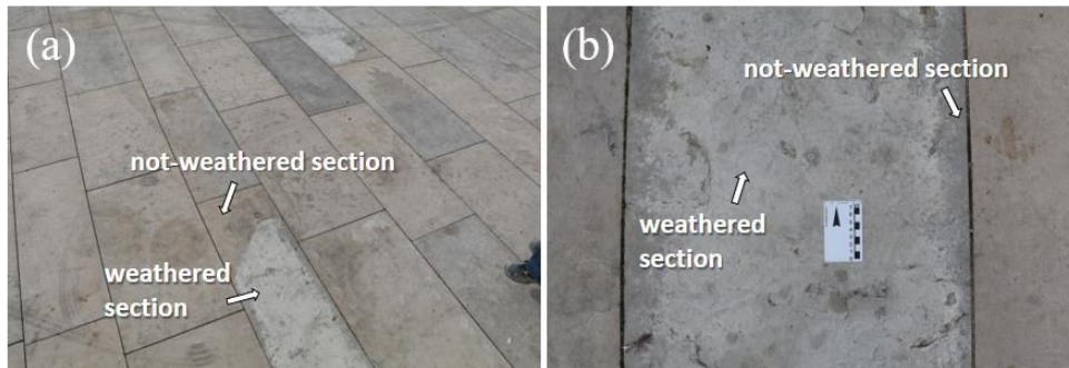
Figure III-2. Building blue limestone with visible alteration (a), (b). ©Luís Lopes
