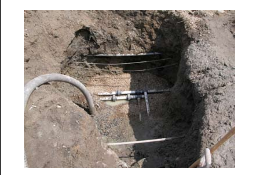
Figure 6. Underground clear water and fertilizer mains, which were cut to show algae and biofilm growth in the absence of sunlight.
