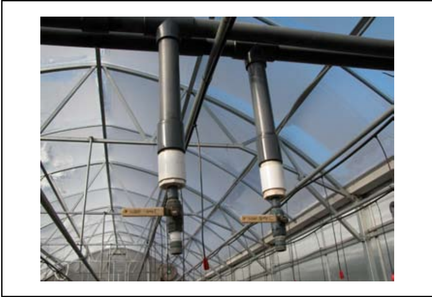
Figure 5. Schedule 80 PVC will not prevent algae growth inside irrigation lines.
