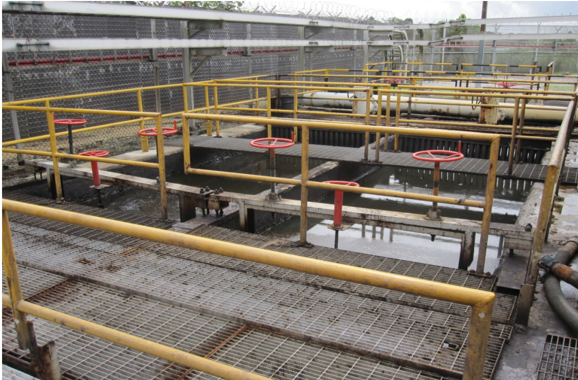
Figure 6: Skimmer Pit used as a Final Produced Water Treatment Step
