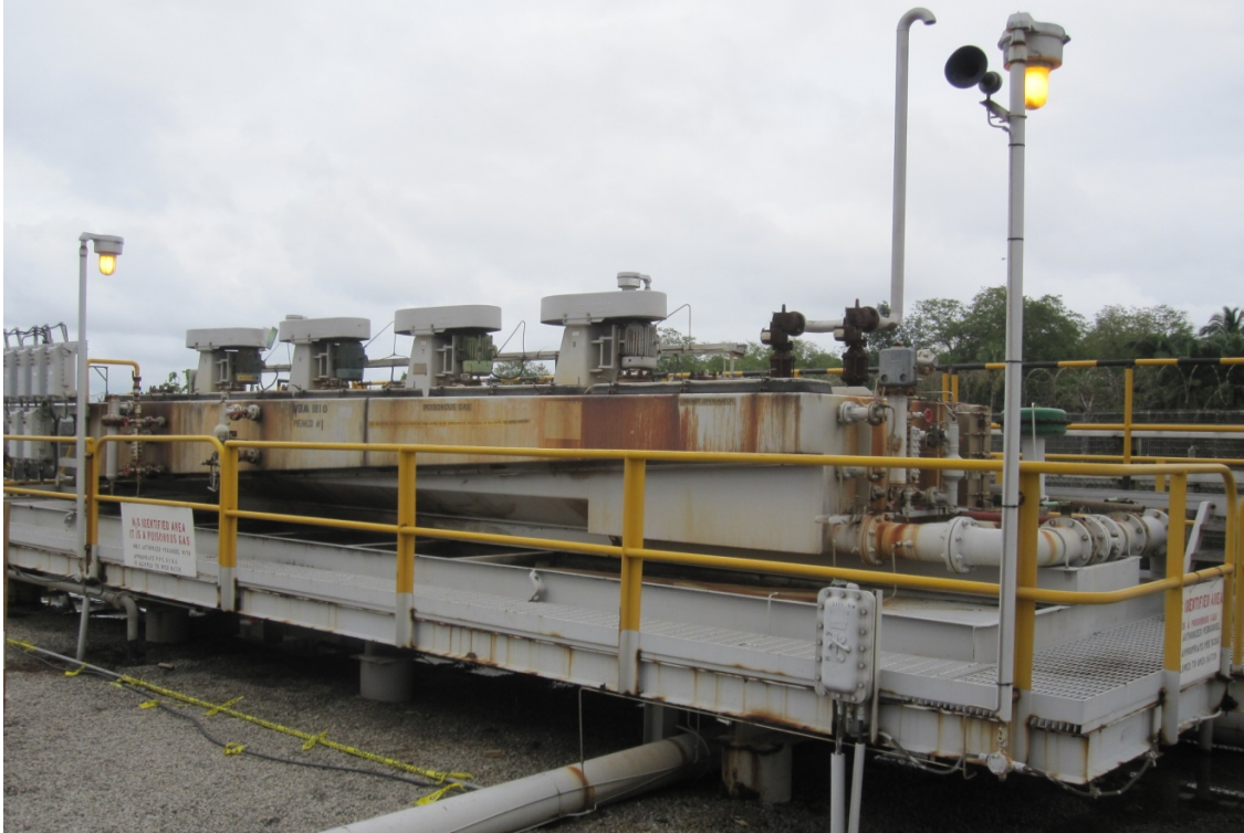
Figure 5: Wemco #1 Unit used during Test A for taking the Samples and Comparing its Performance with Enviro-cell Unit
