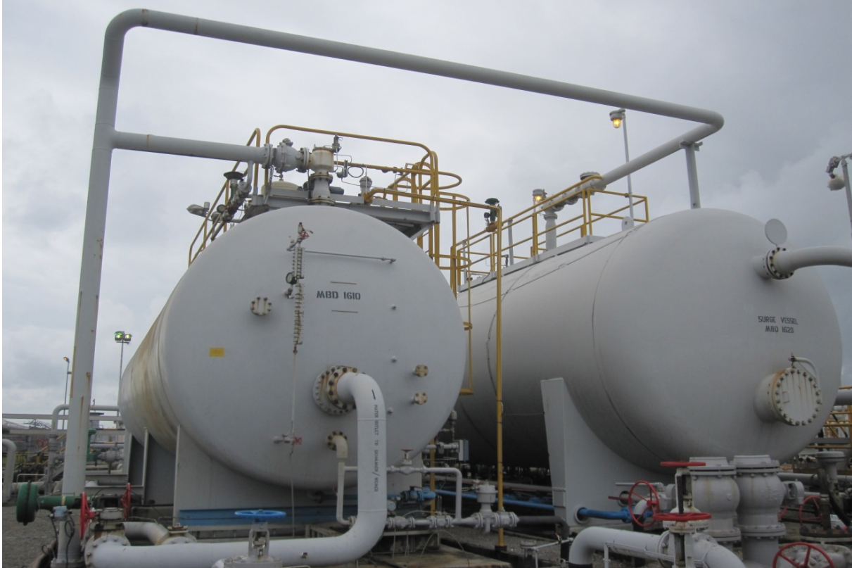
Figure 4: Surge Vessel before the Enviro-cell Pilot Unit and Wemco Unit for Secondary Oil Separation
