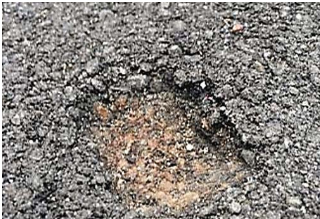
Figure 3. A 5 cm x 5 cm (2-inch by 2-inch) crater or miniature pothole, 2.5 cm (1-inch) deep is formed during the month of October 2014, resulting from a 880 N. (200 lbf) load applied over a 30-day period
