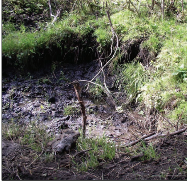
Photo 2.7 - Top of Shorty Creek showing vertical instability in the form of a headcut.
