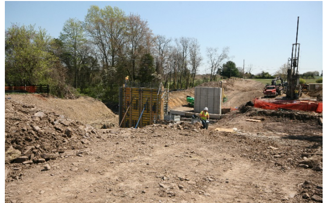
Figure 3-15: Current work on the site of the truss bridge. Steel structure will be returned after construction. Source: CHG
