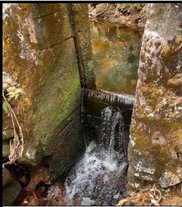
Sluice gate in disrepair returning ditch water to Kawaikōi Stream
