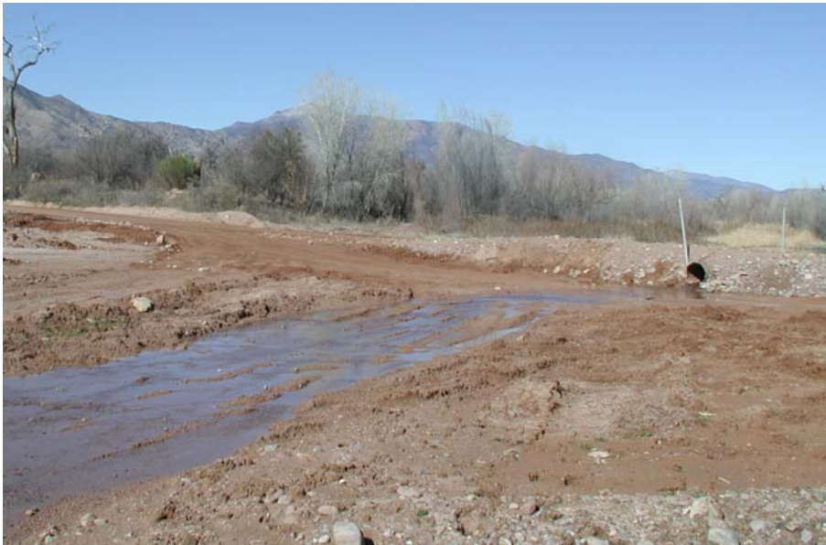
Plate 4- The A-Cross Road Low-water ford. (Example of periodic decline in water quality as a result of low-water fords)
