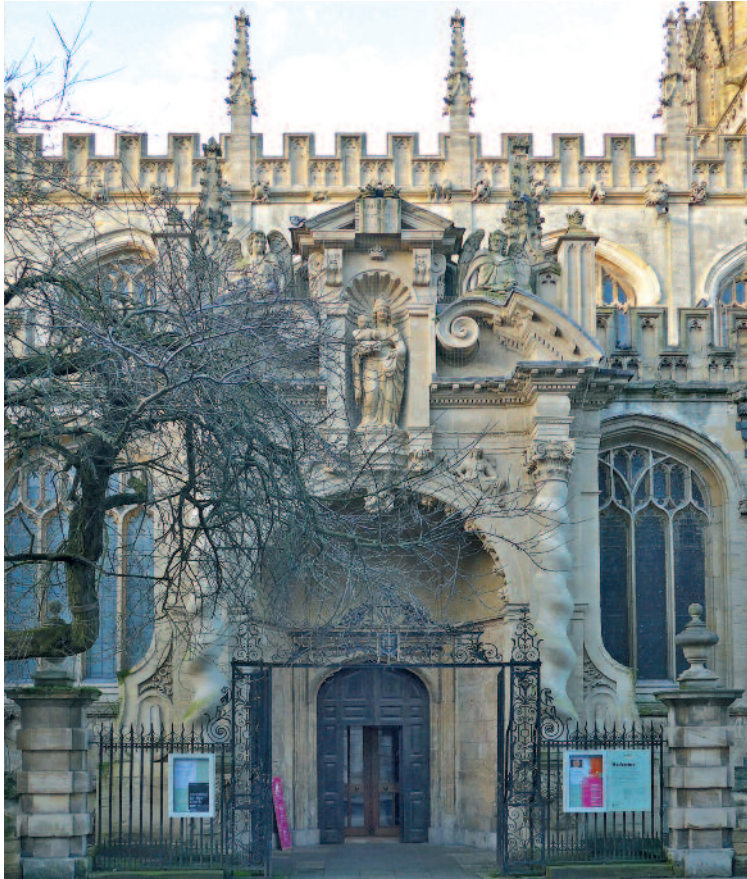
Fig. 4. The porch of St Mary the Virgin, Oxford (1637), showing the buttresses – the upper part is partly obscured by a protected tree. ( Silvia Maiorino , 2015)
