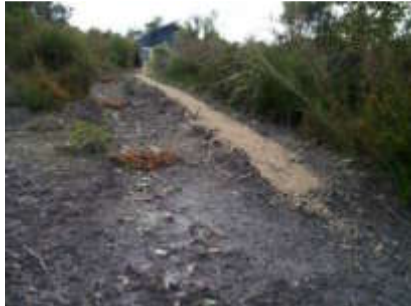
Stormwater directed from private property onto the Reserve at Springdale Heights
