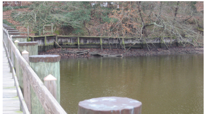
Timber bulkhead with base sediment accumulation visible at low tide in Talbot County. (Rebecca Swerida)
