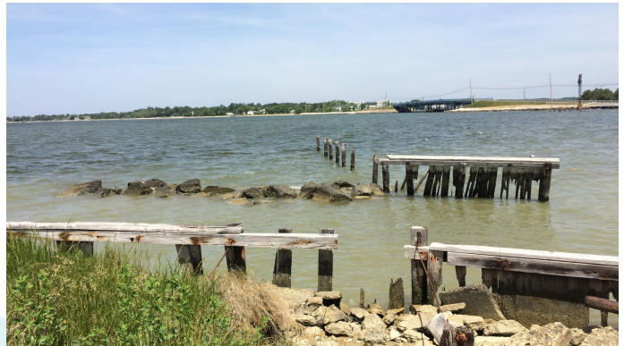
A very complex shoreline in St. Mary's County contains several failed shoreline control structures cannot be effectively categorized. (Rebecca Swerida)
