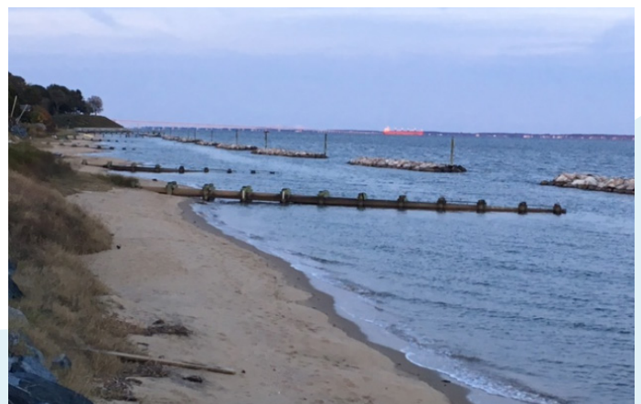
Large off-shore stone breakwater structures paired with timber groins in Anne Arundel county. (Rebecca Swerida)
