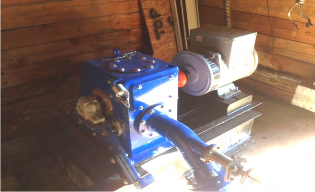
New Turbine and Generator
