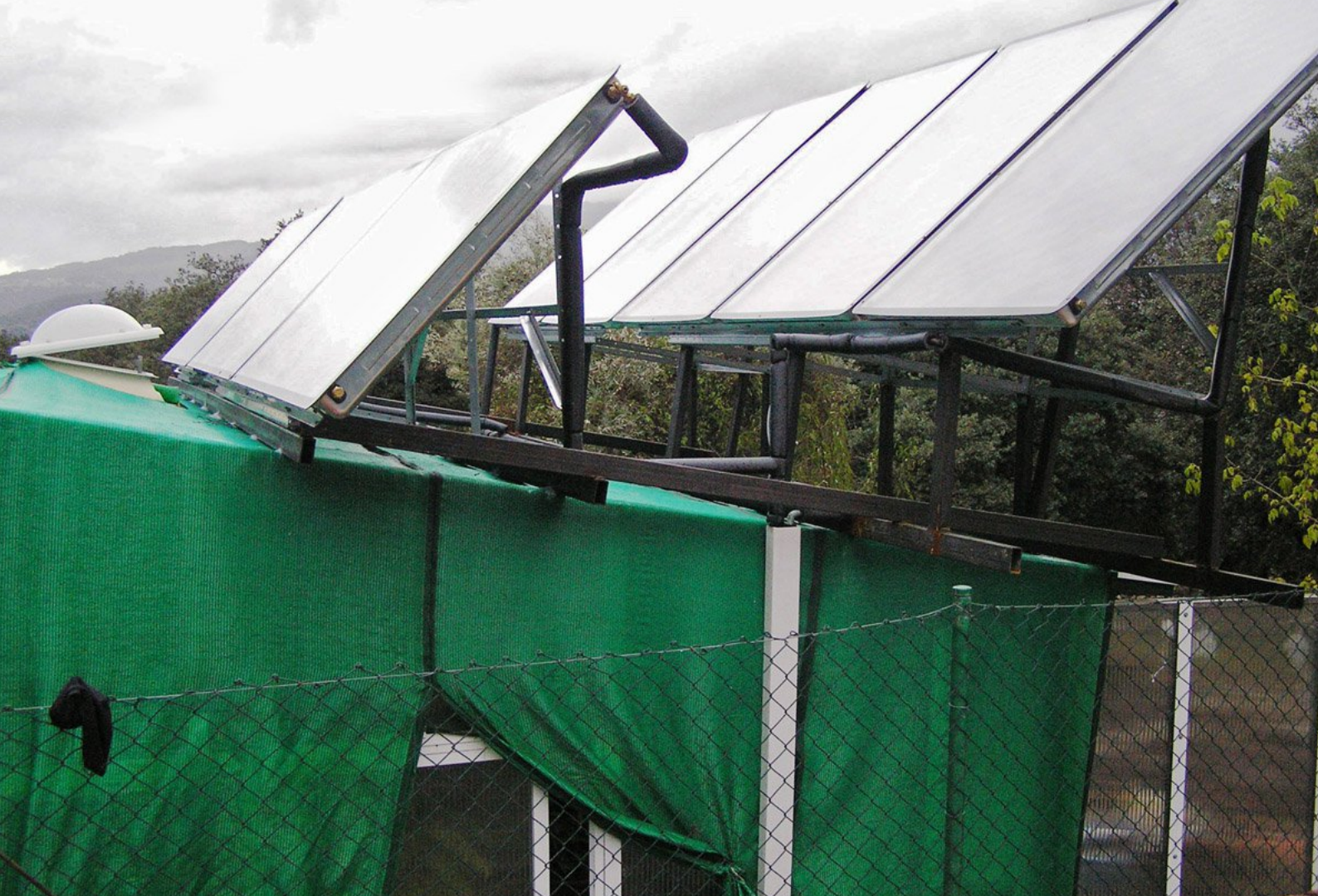
The double array of solar panels installed to heat the greenhouse.
