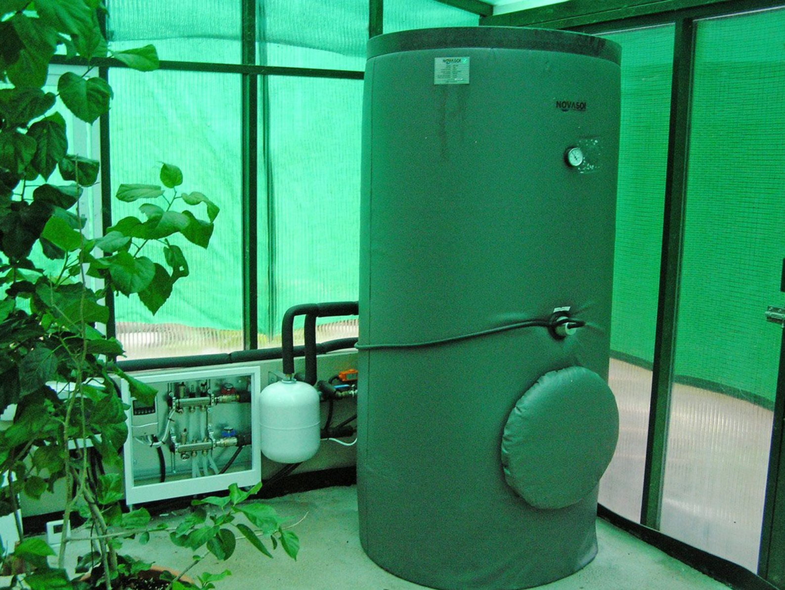
The water storage tank and pump which pipes warm water under the new floor of the greenhouse.
