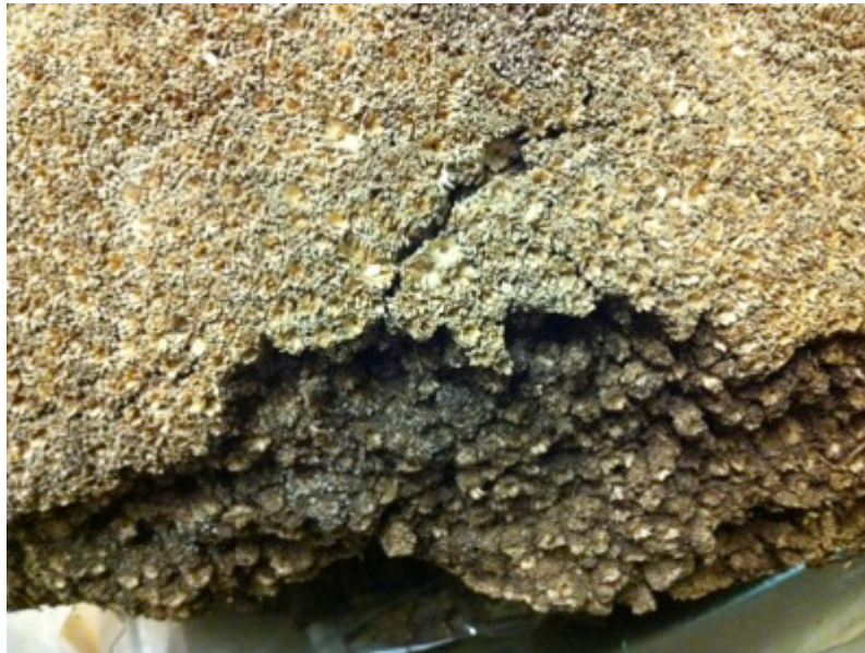
Loss of material at base
