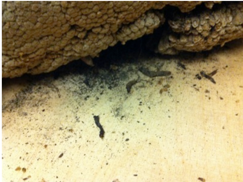
Debris at base
