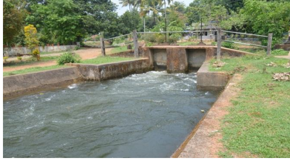
Left Bank Main canal (Regulator at Palissery)
