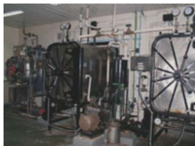
Barrier (double door) autoclaves, one door opens in containment area.
