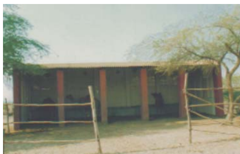
Shed with asbestos roof
