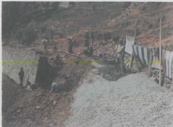
Site of construction for staff quarter at R/S Bhowali is in progress.
