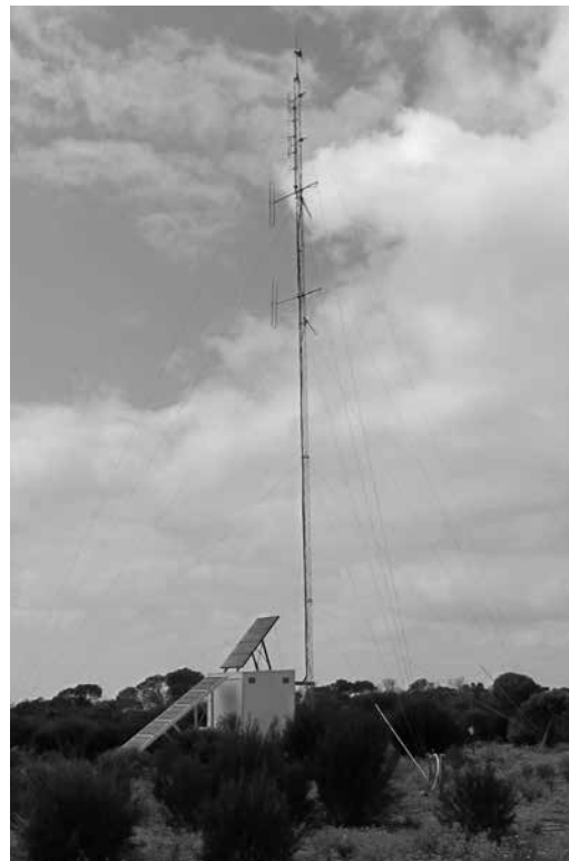
Police and DPaW radio communication repeater station and tower on Meanarra Hill. Photo – Mike Paxman (DPaW)
