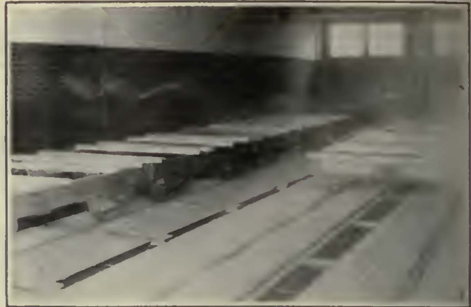
Interior of Dry Lumber Kiln Showing the Tracks, Gratings and Ventilating Arrangement
