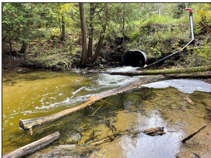
Undersized culvert on Spirit Creek at Lake Shore Drive.
