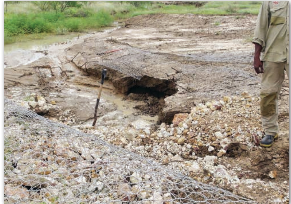
Subsequent scouring of remediated erosion area.
