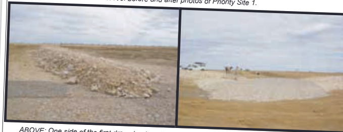
ABOVE: One side of the first drop structure (partially complete) down from the culvert and the wire armoring to the apron opening
