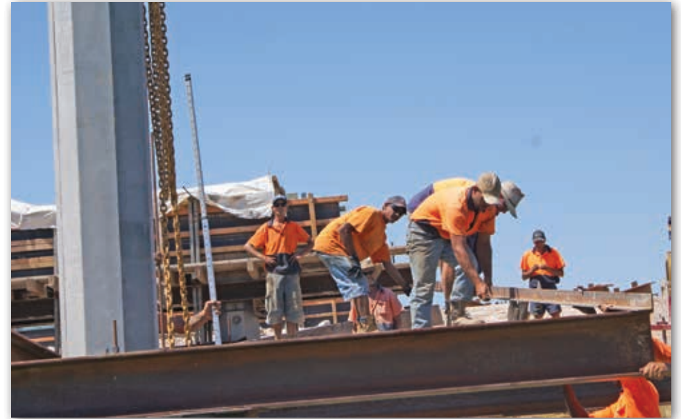
Young Ganalidda men - Trinity Yanner and Warick Walden working on the new Gumbumunda Bridge in Burketown.
