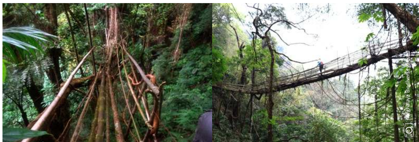
Under construction living root bridge (about 52 m long) Mawkymnot village near Pynursla.
