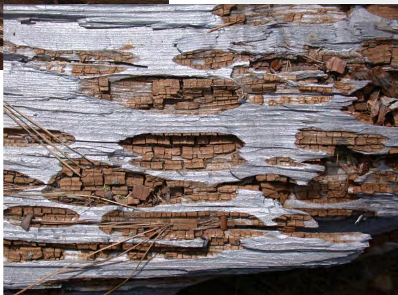
Damage from dry pocket rot. Photo: Darvin DeShazer.
