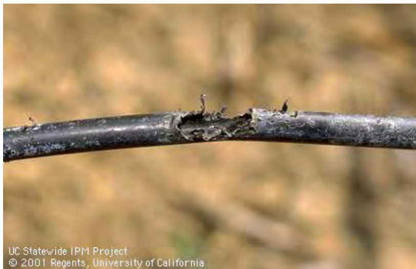
Ground squirrel damage to an irrigation line. Photo: Jack Kelly Clark/UC IPM.
