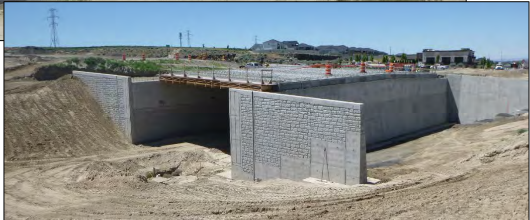
US395 interchange project that will provide full access to Ridgeline Drive is currently under construction.
