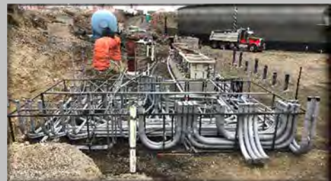
Reservoir Pump Station
