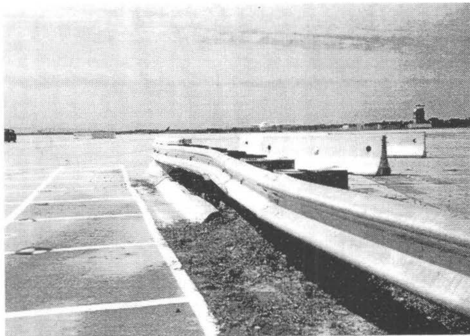
FIGURE 23. PHOTOGRAPHS OF DAMAGE TO APPROACH GUARDRAIL TRANSITION SECTION.
