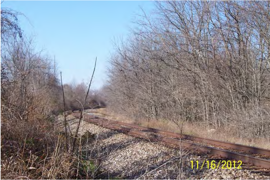
Photo 28: 1° 34' Curve at MP 344.5 west of Columbia City, there is a ravine on the inside of this curve.
