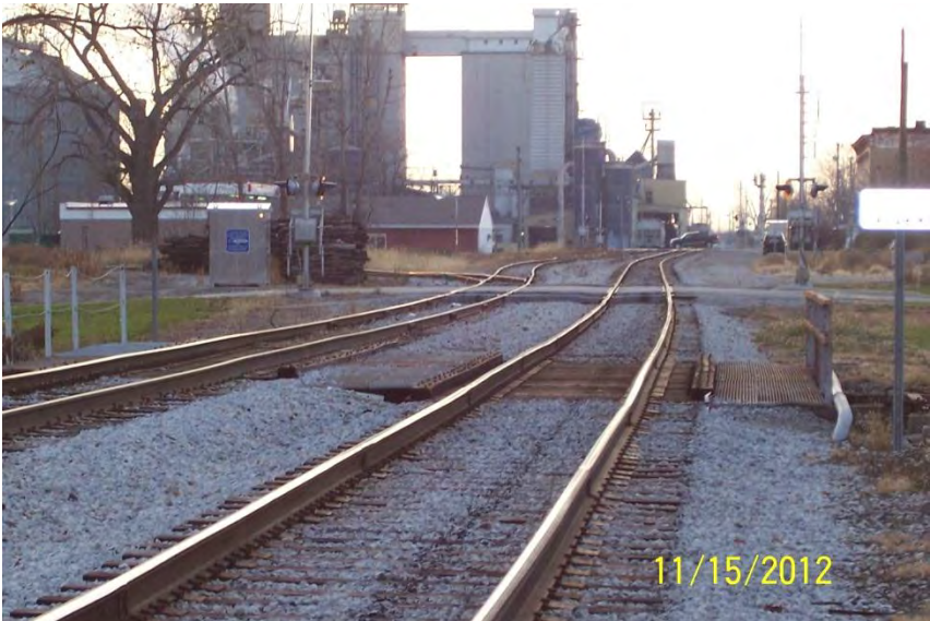
Photo 16: The main track alignment needs straightening in Delphos, OH
