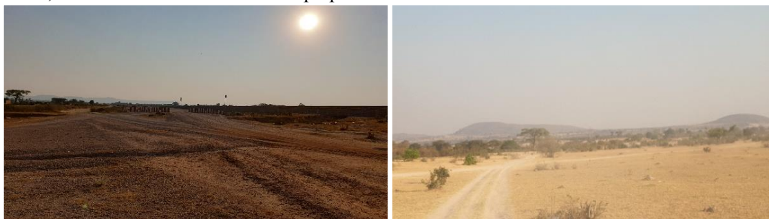
Figure 7.7-14 Paved (left) and unpaved (right) roads in need of repair in Lubango
