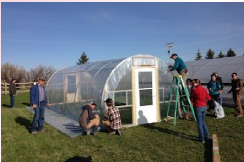
THG Summer Practicum students along with Mac Burgess and David Baumbauer replacing polyfilm on a small high tunnel.
