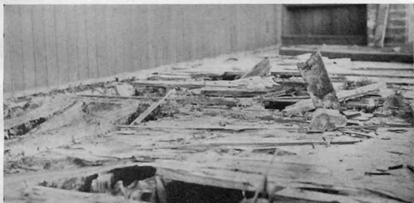
b. Rotten Condition of Living Room Floor.
