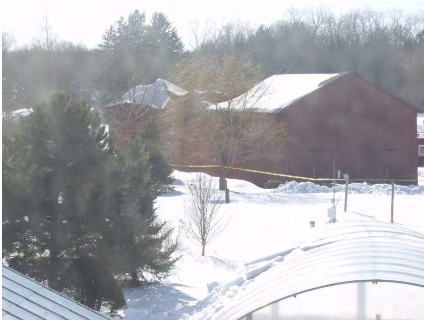
Tobacco shed roof collapse during winter 2011.
