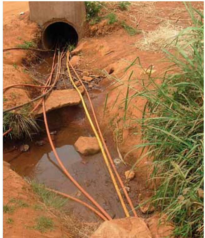
Irrigation pipes in the highlands of Bafou (near Bamboutos Mountains). Photo: © J.P. Ghogue.
