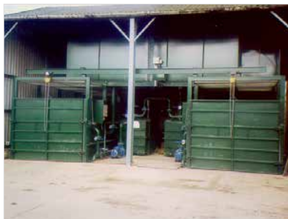
48 Typical front-loading HWT equipment with common holding tank above
