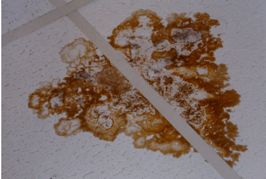
Fig. 6. Typical ceiling tile leak colonization by Alternaria ( Ulocladium type) and Penicillium .
