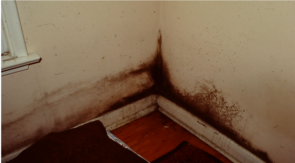
Fig. 1. Cladosporium mould on a poorly insulated wall, with moisture produced by condensation in cold outdoor weather and lack of air circulation due to furniture (bed) against the wall.
