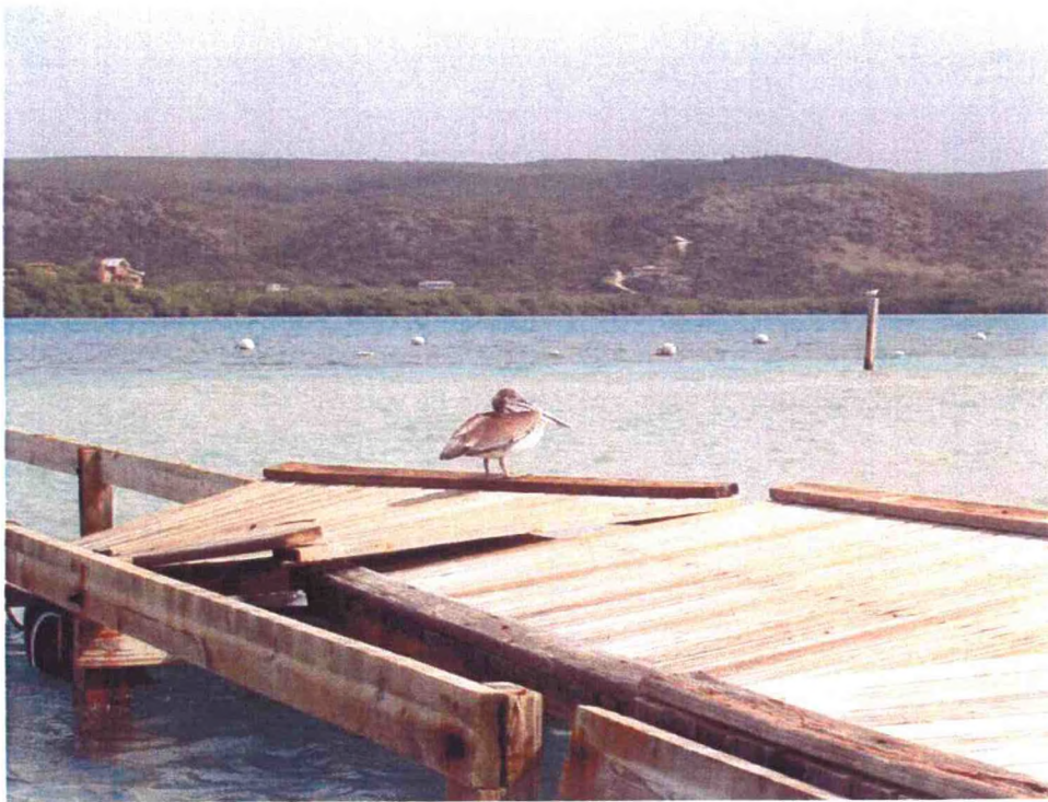
Plate 2. Damage to DNER infrastructure by Hurricane Ivan in September 2004.
