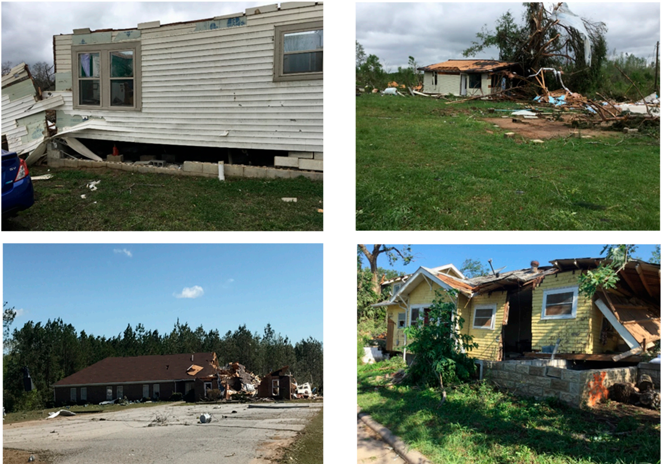
Figure 8. Damages (DoD = 5, entire house shifts off foundation) on one- or two-family residence under EF = 2 as would ideally correspond to a “considerable” impact tag. All images were retrieved from NWS damage assessment toolkit [68].
