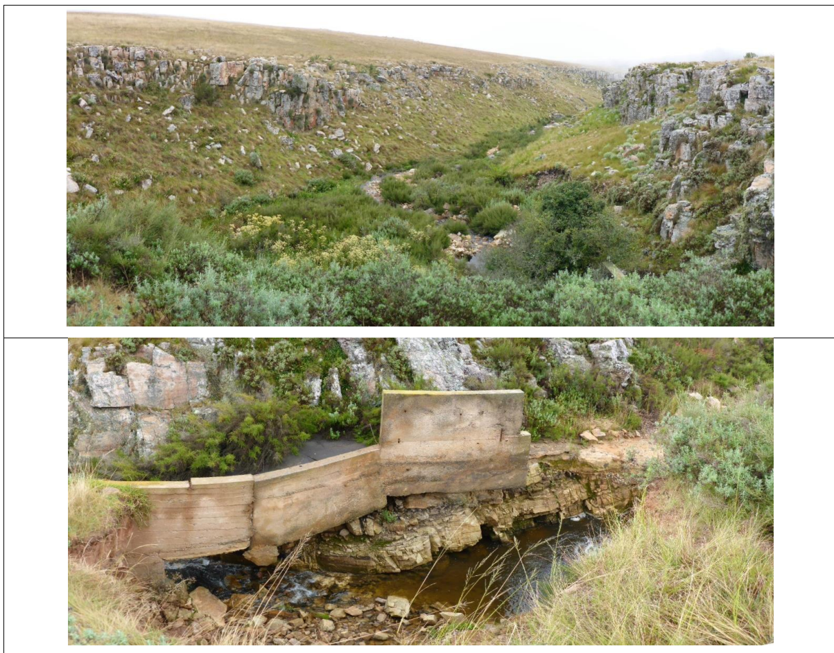
Figure 12: Illustrates an intact mountain stream (BMU 7) with a bedrock channel bed located directly downstream of an eroded dam spillway.
