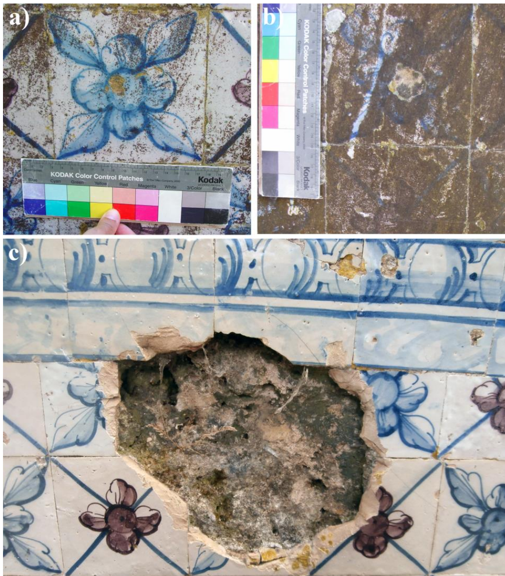
Fig. 6.1. Images damage and different pathologies found on the Casa da Pesca glazed wall tiles. (a) brown biological colonization, lacunar and detachment of the glaze; (b) severe biological colonization and lacunae of the glaze; and (c) biological colonization, lacunae of tiles and mechanical damage due to theft or vandalism.
