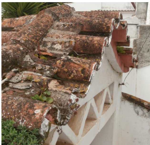
Fig. 2.5. Biological colonization of roofing tiles from a house in Alentejo region (south of Portugal).
