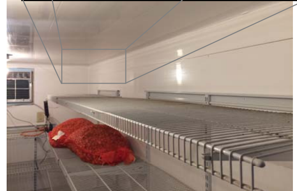
A properly outfitted cooler results in a clean install both visually, and physically. Note the use of trim pieces to close gaps at corners.
