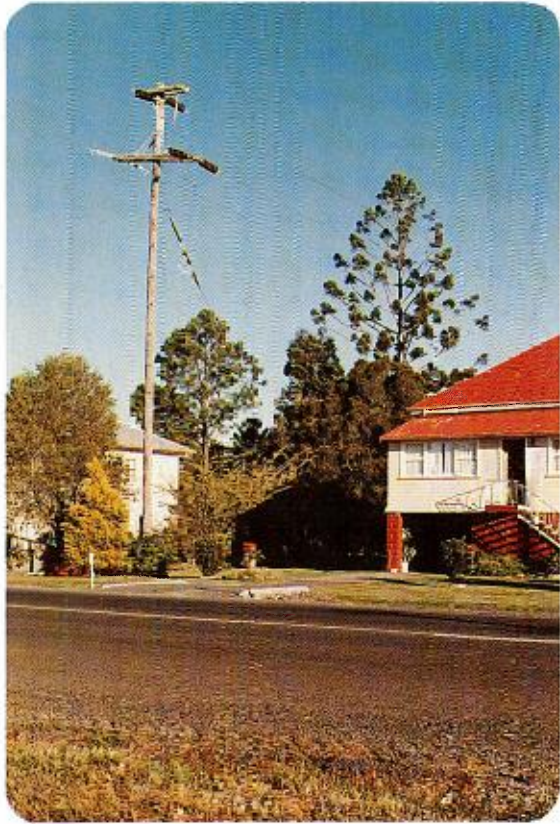
Existing 66 kV line crossing Casino Street
