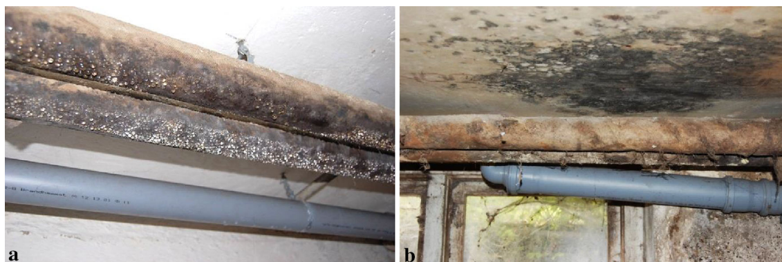
Fig. 9 Stachybotrys a growing on water saturated pipe insulation due to a leaking pipe (water drops can be seen hanging from the insulation), b on gypsum ceiling tiles after severe condensation in a basement
