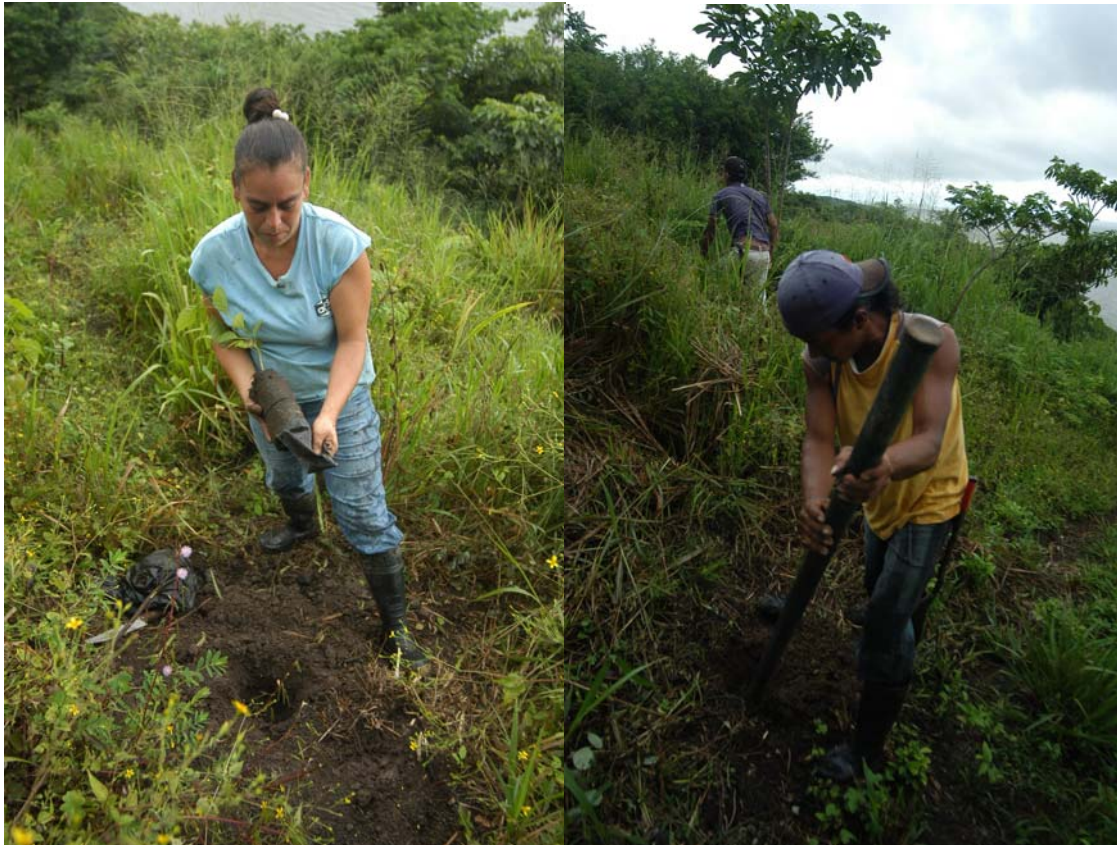
Figure 31. Community workers digging holes and placing trees in the ground at reforestation site.
