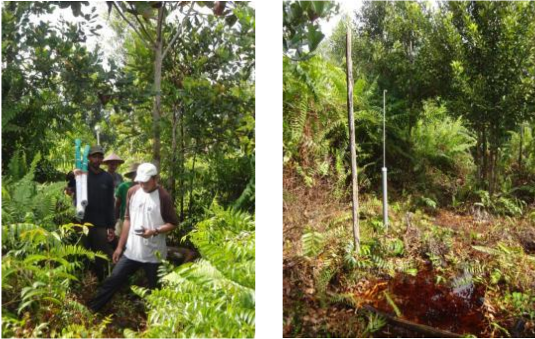
Figure 28 Installation of tubewells for monitoring of ground water levels in project area
