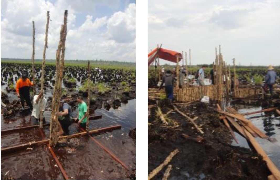
Figure 20 Construction of a simple dam in the Timba canal of Rasau watershed
