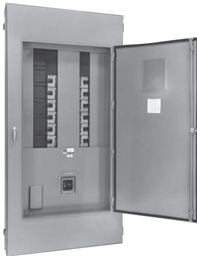
Access to Circuit Breaker Handles
