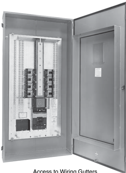
Access to Wiring Gutters
