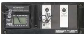
Electronic Trip Unit with Seals Installed to Restrict Access
